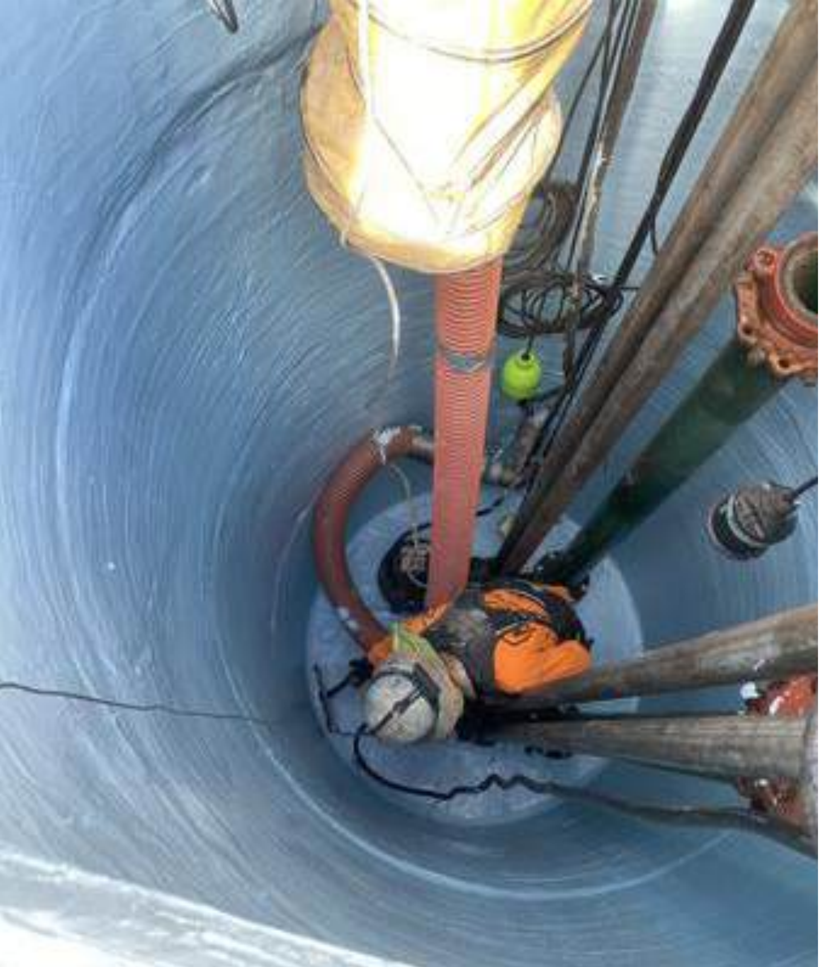
Lift station upgrade—enhancing capacity, reliability, and long-term performance of the wastewater system.
