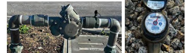
Examples of a backflow device (below) and a water meter (right).
