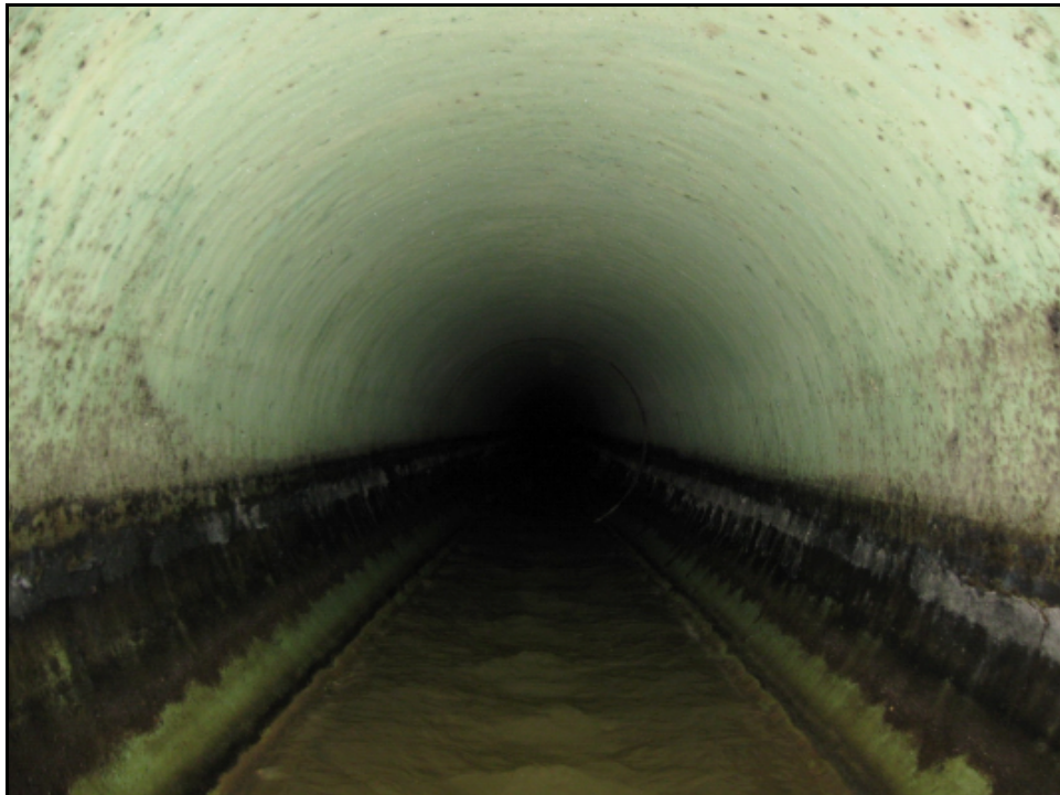
North Influent Pipe
