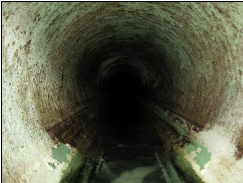
North Influent Pipe
