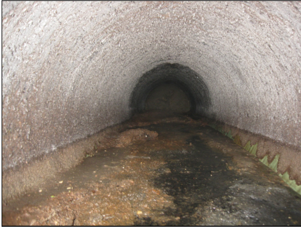
East Plugged Pipe
