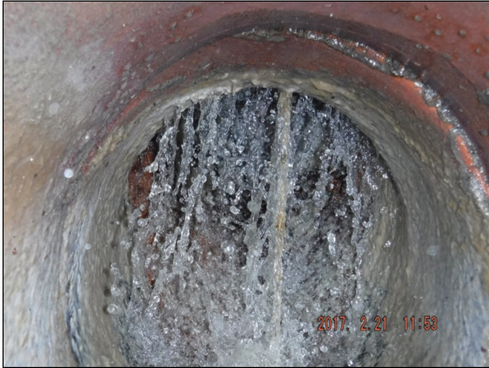
Lower Influent Pipe
