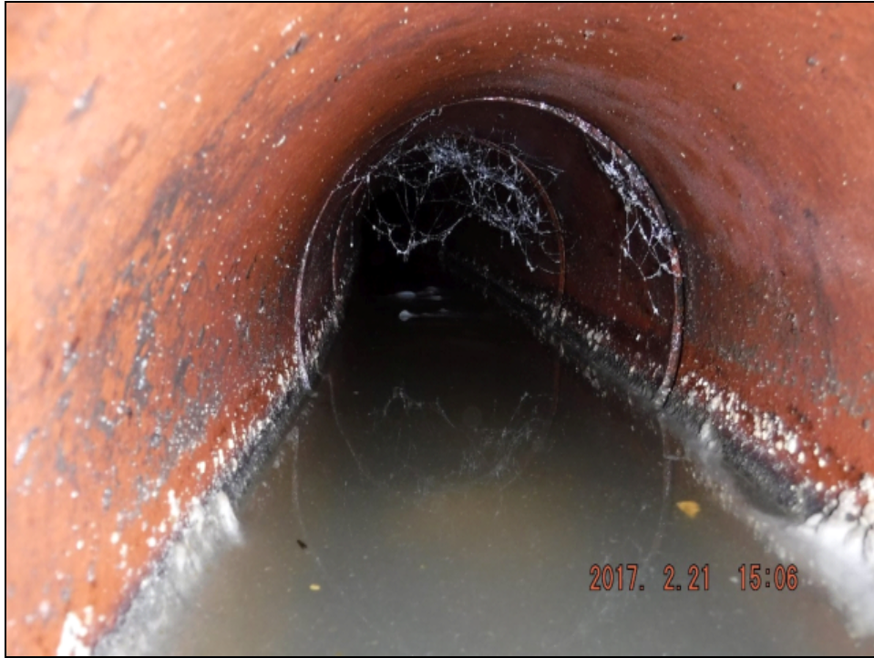
West Influent Pipe
