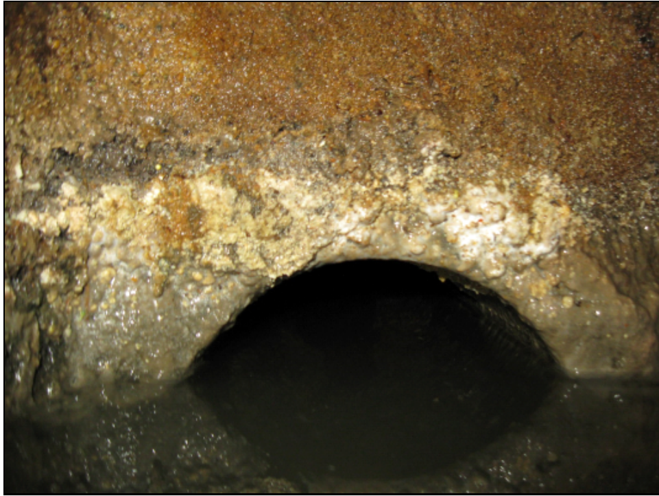
South Influent Pipe
