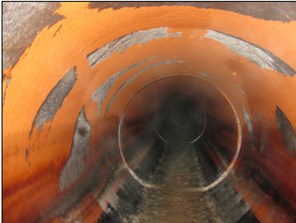
South Influent Pipe
