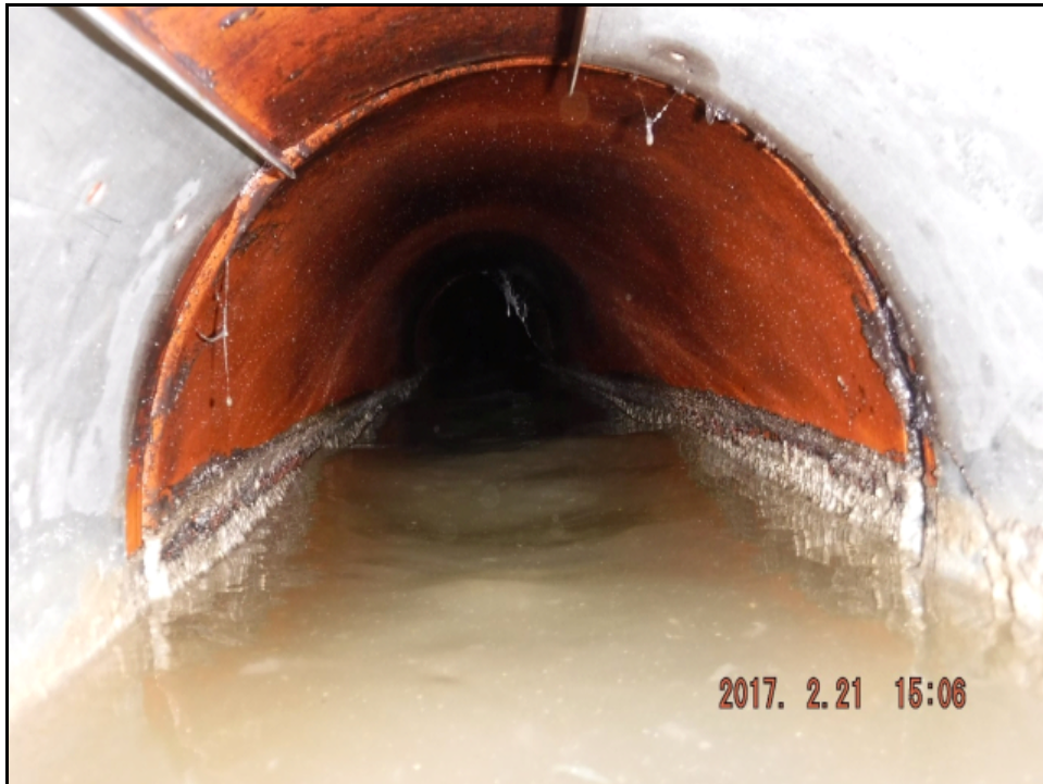
South Influent Pipe
