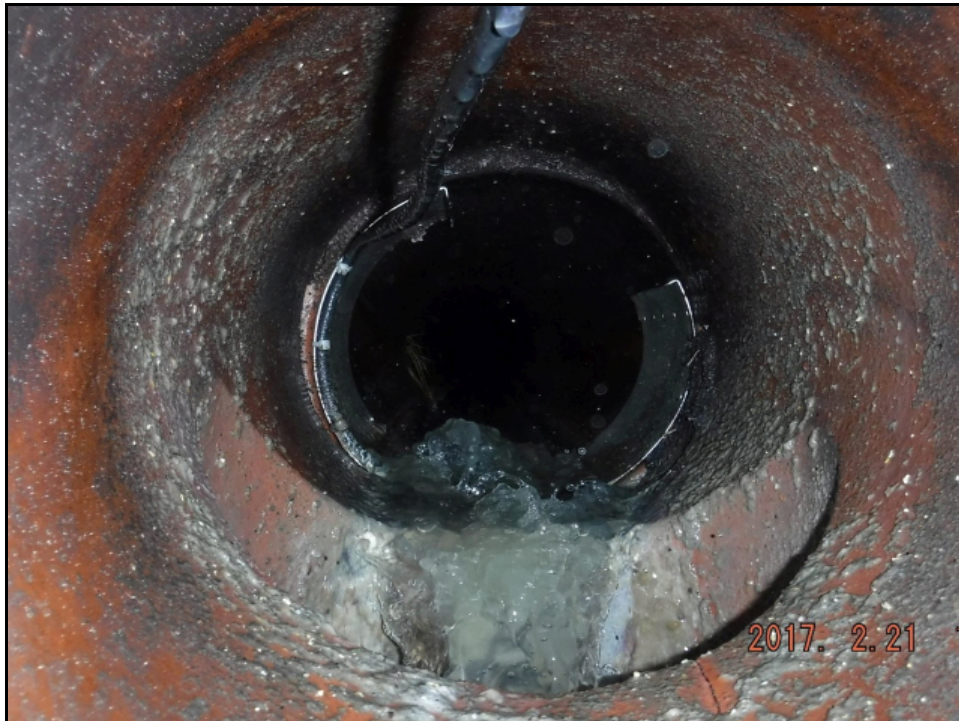
Upper Influent Pipe
