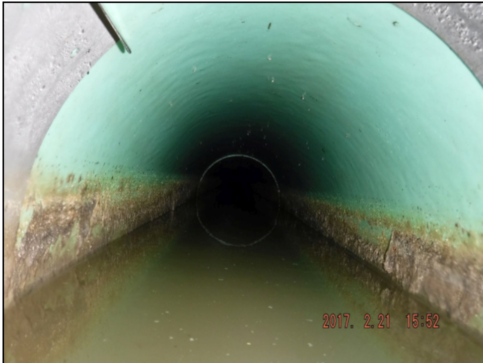
West Influent Pipe
